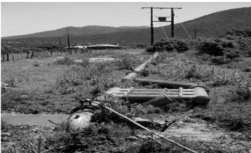
Figure 5.2: Example of block off take showing flow metre, pressure gauge, filters, non-return valve and electrical supply for booster pumps
